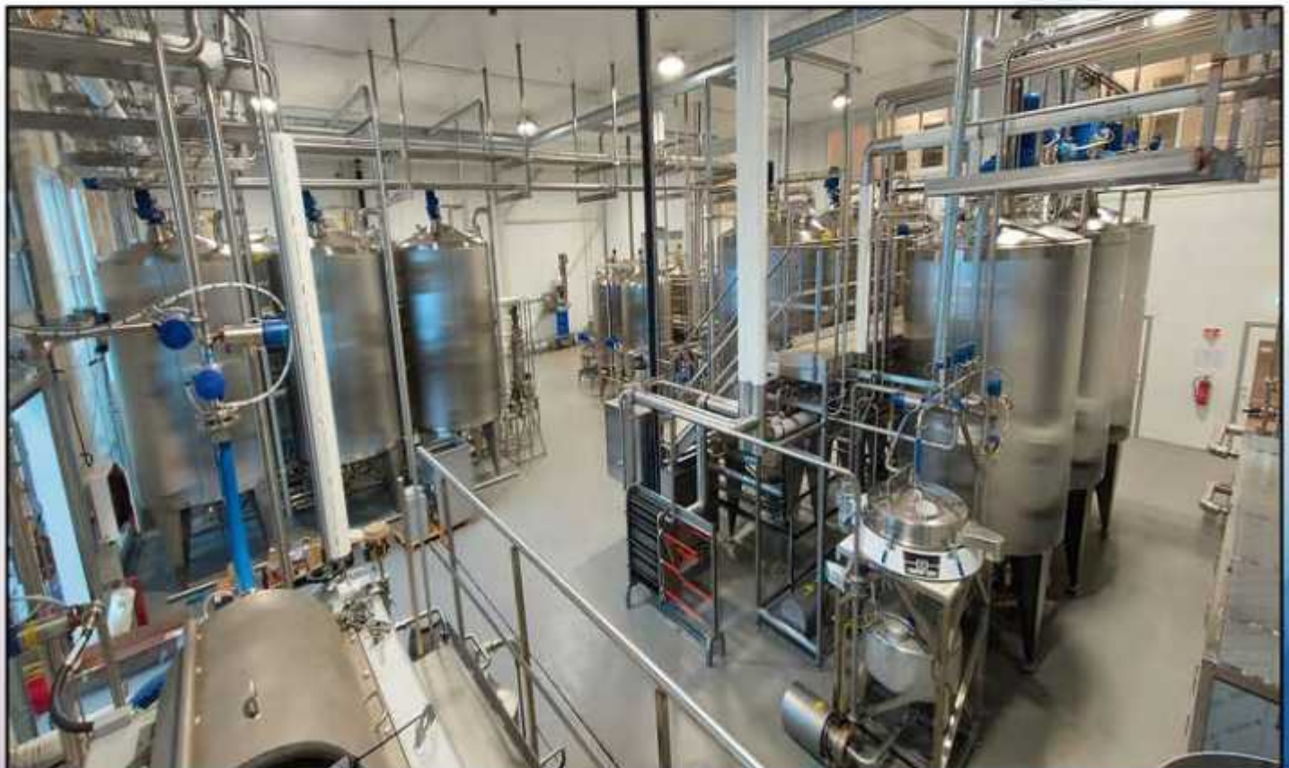
Fig. 3. The Zoooca Process Plant Tromsøe Norway
